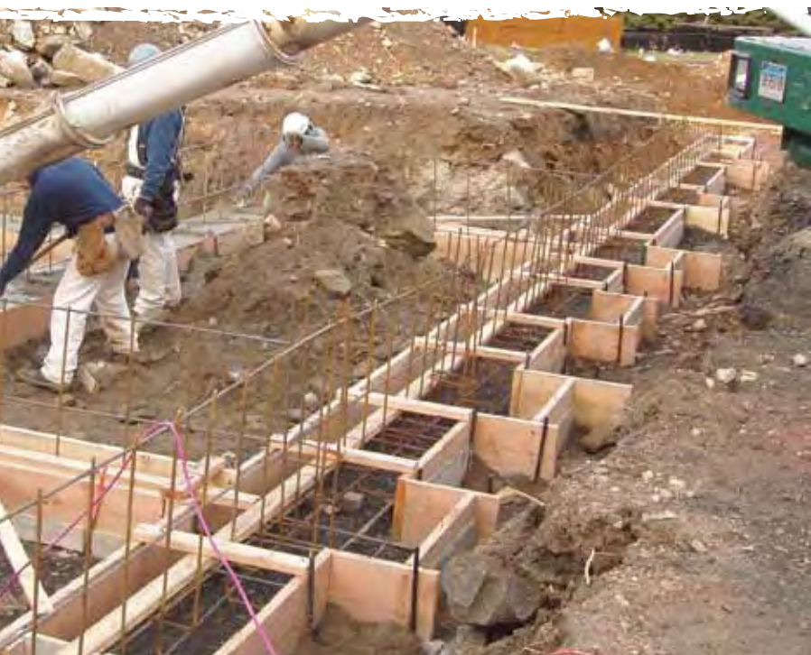
Figure 5 Pier footing with sides running wild
